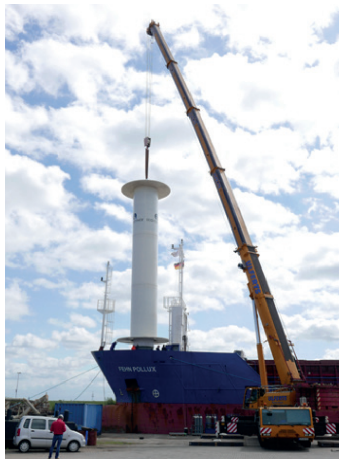
Installation of a Flettner rotor prototype on the Fehn Pollux as part of a reallab
